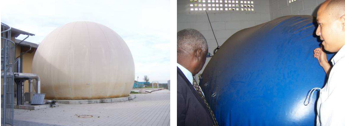
Figure 7.26 External low pressure gas storage tanks (RUTZ 2007)
