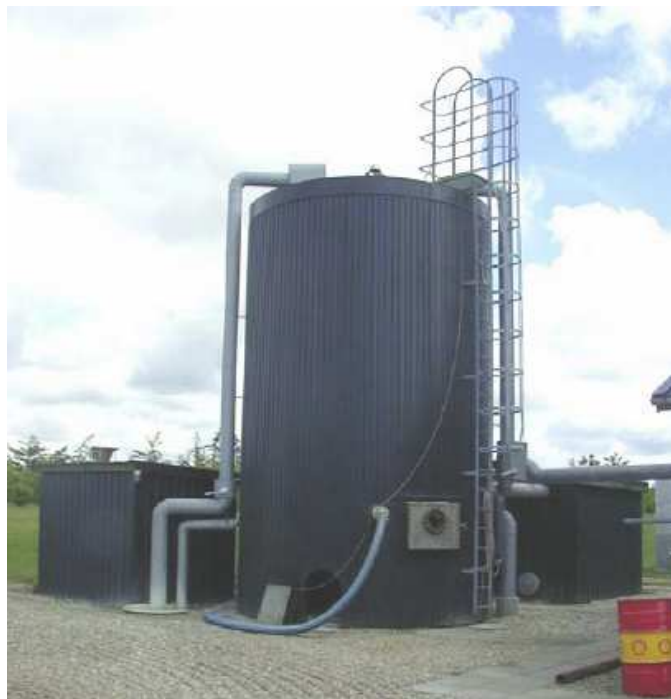
Figure 7.31 Reactor tank for removal of hydrogen sulphide (ANGELIDAKI 2004)
