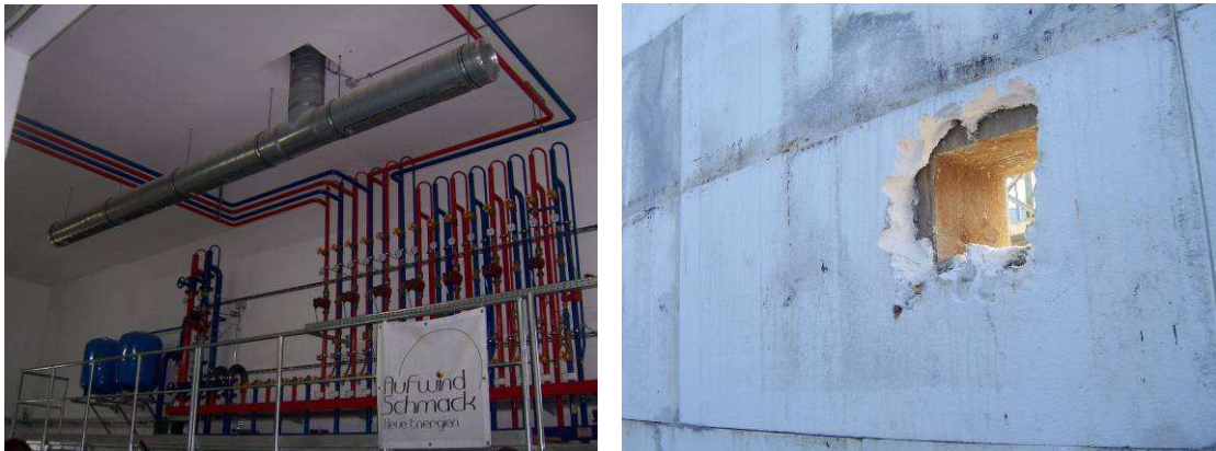
Figure 7.16 Heating system of a biogas plant ( left ) and insulation of a concrete digester, under construction ( right ) (RUTZ 2008)
