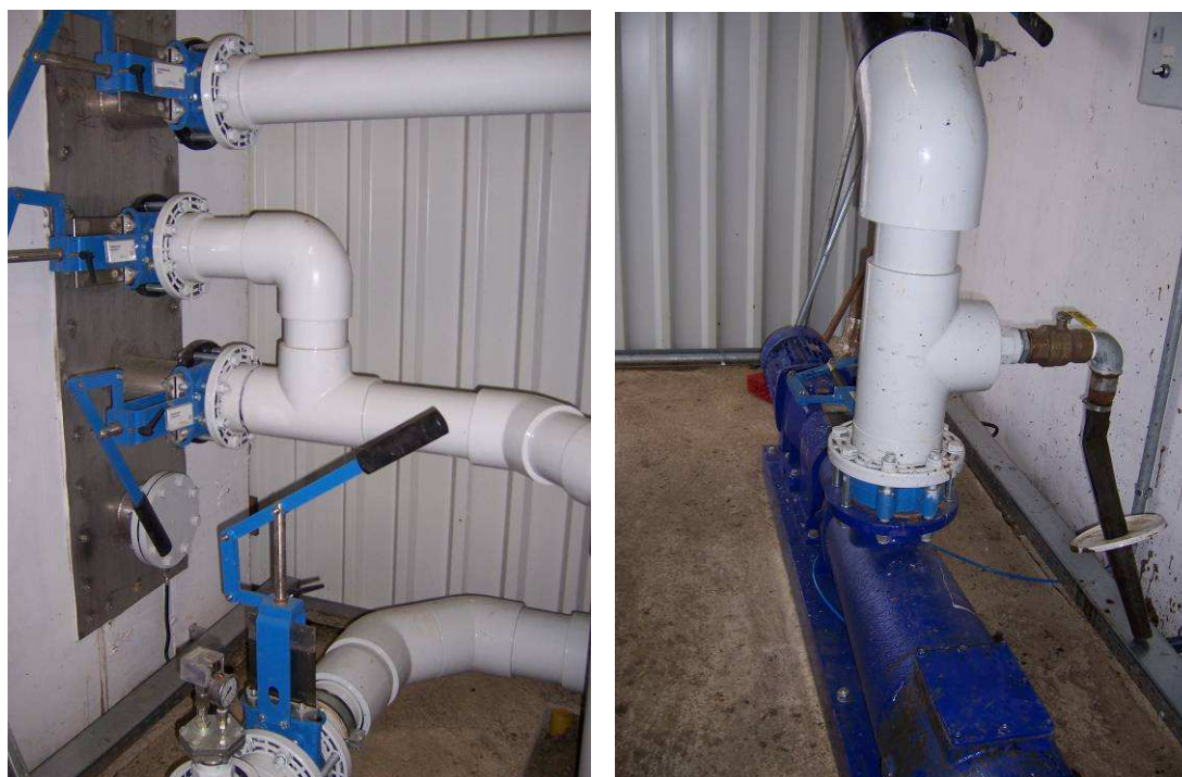
Figure 7.8 Stop-valves ( left ) and pumping system ( right ) (RUTZ 2006)
