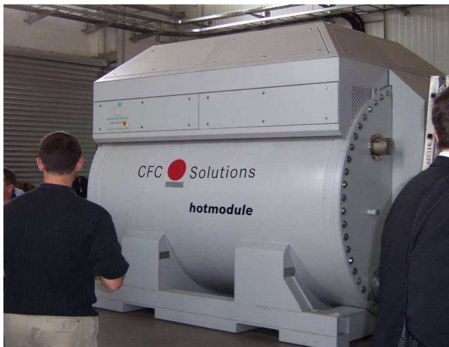
Figure 5.6 World's first MCFC fuel cell for biogas, operating in Germany (RUTZ 2007)
