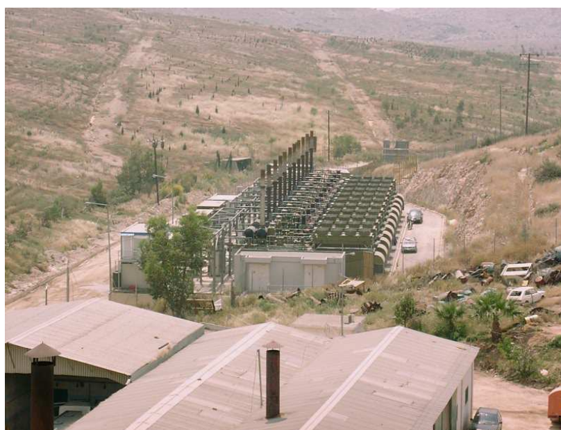
Figure 4.14 Ano Liosia Landfill gas exploitation project, Athens, Greece
