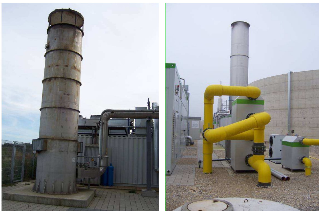
Figure 7.28 Modern biogas flares (RUTZ 2007)
