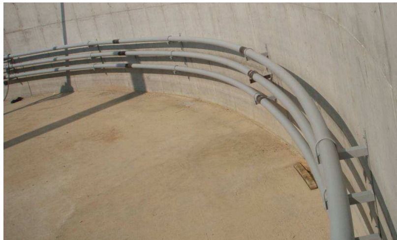
Figure 7.17 Heating pipes, installed inside the digester (AGRINZ 2008)
