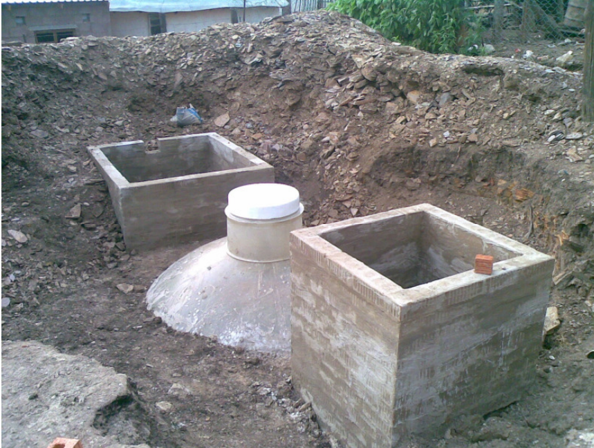
Figure 14: Construction shot of household digester for processing cattle manure, biogas produced fully offsetting fuel wood use and providing much needed fertiliser in the form of bioslurry to the garden (Source: AGAMA Energy, 2008).
