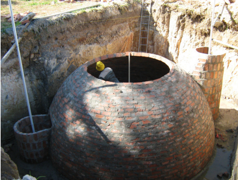
Figure 12: Construction of a 20m 3 biogas digester for processing sewage wastewater, food scraps and chicken litter (Source: AGAMA Biogas, 2007)
