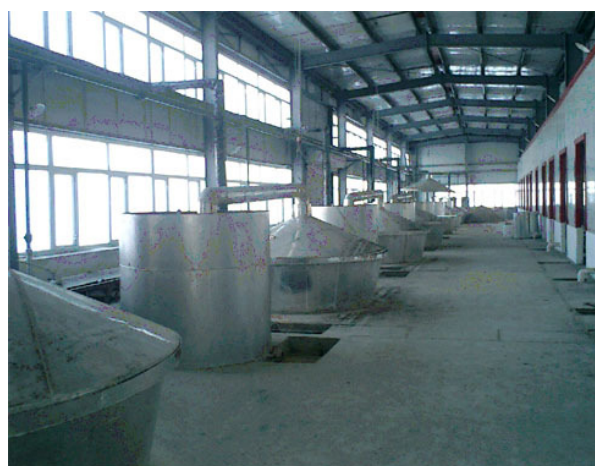
Brut distillation workshop of making fuel ethanol
