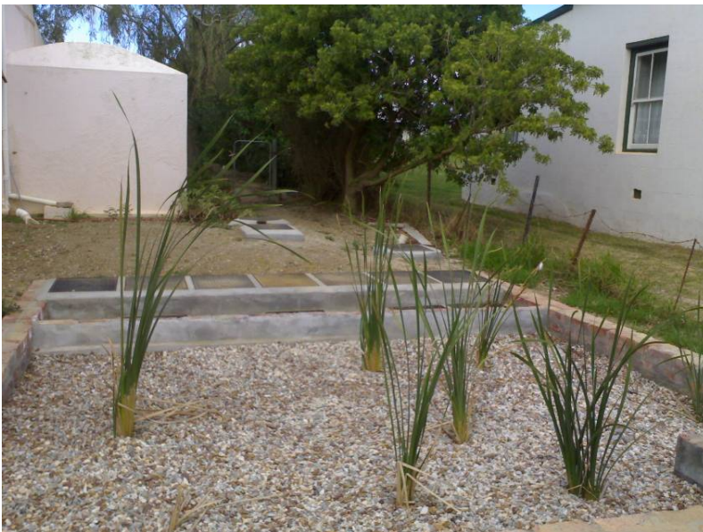
Figure 13: 4m 3 single household digester (in background), anaerobic baffled reactor (midground) and gravel filter (foreground) producing water from processing sewage and food scraps to produce thermal energy for cooking and water that is compliant water quality standards (Source: AGAMA Biogas, 2007)
