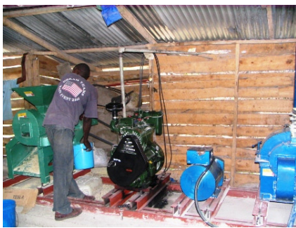
MFP plant installed at Leguruki
